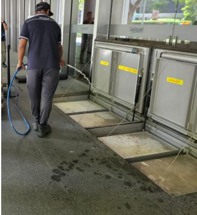
Flood barriers at CapitaSpring that pop up for flood prevention into the building
